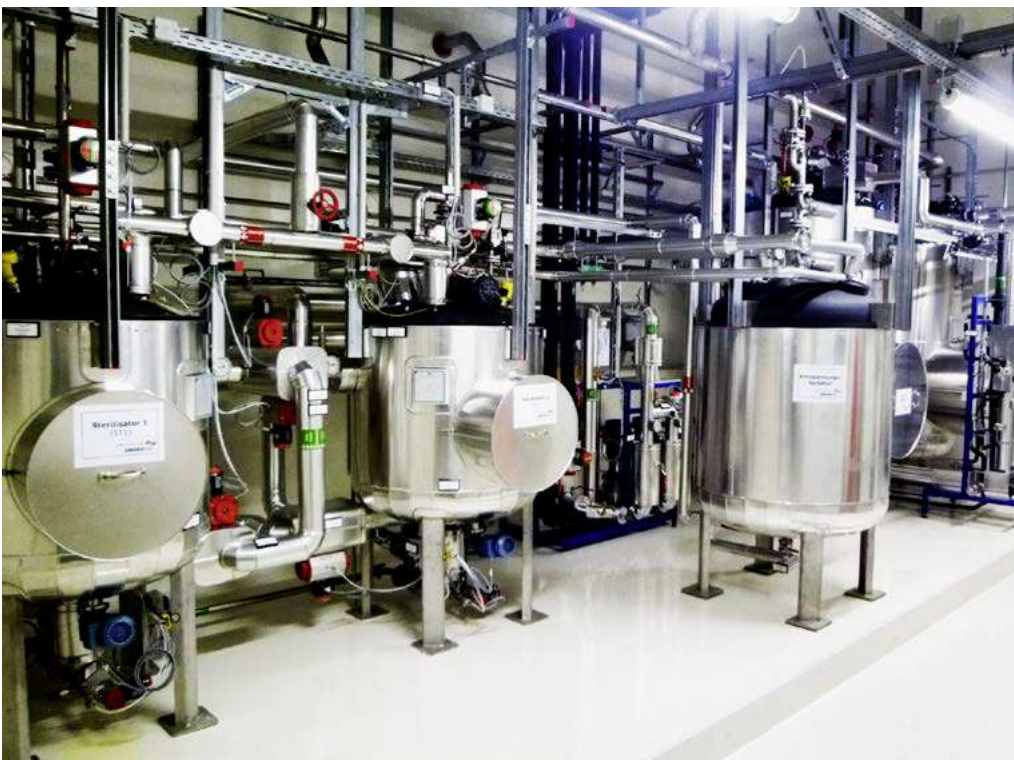
Wastewater treatment facility
